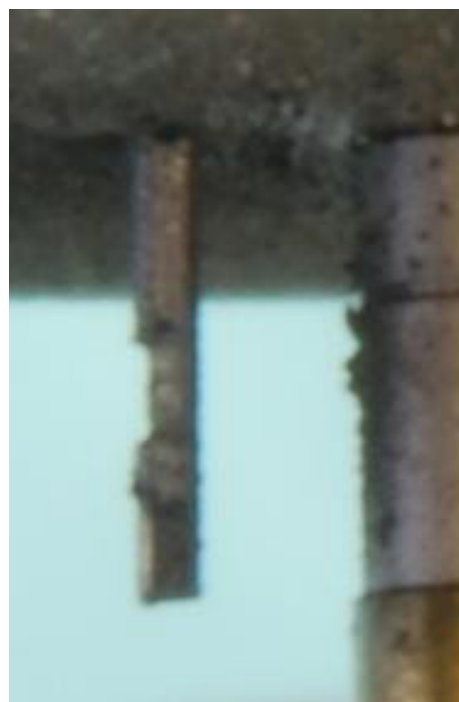
This pin is about 50% burnt through by many millions of sparks..
